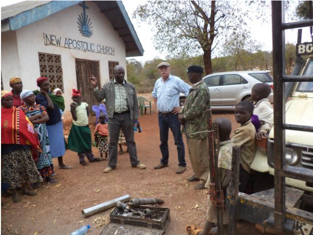
Removal of Broken Pipes was attempted by Testek in July '12
