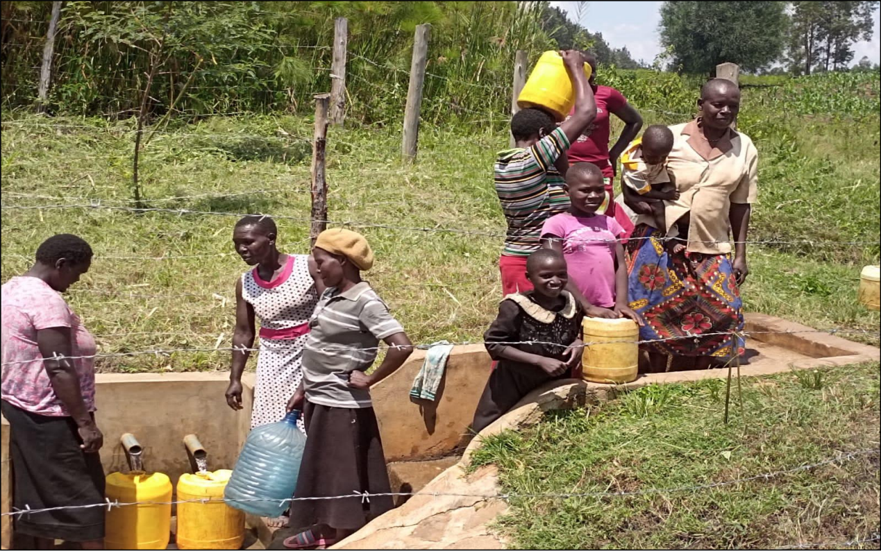
9.0 Women Community members fetching water from Kibachenje spring protected and constructed by KUMEA
