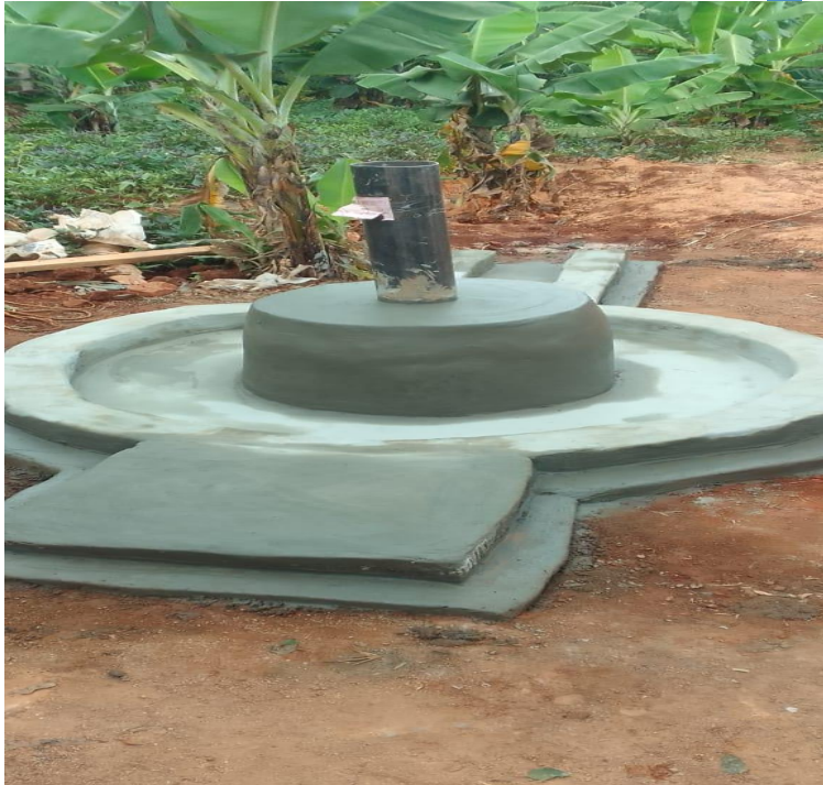
7.0 Completed Imonyelo Self Help Group Hand dug well in Mungona location of Vihiga Sub-county
