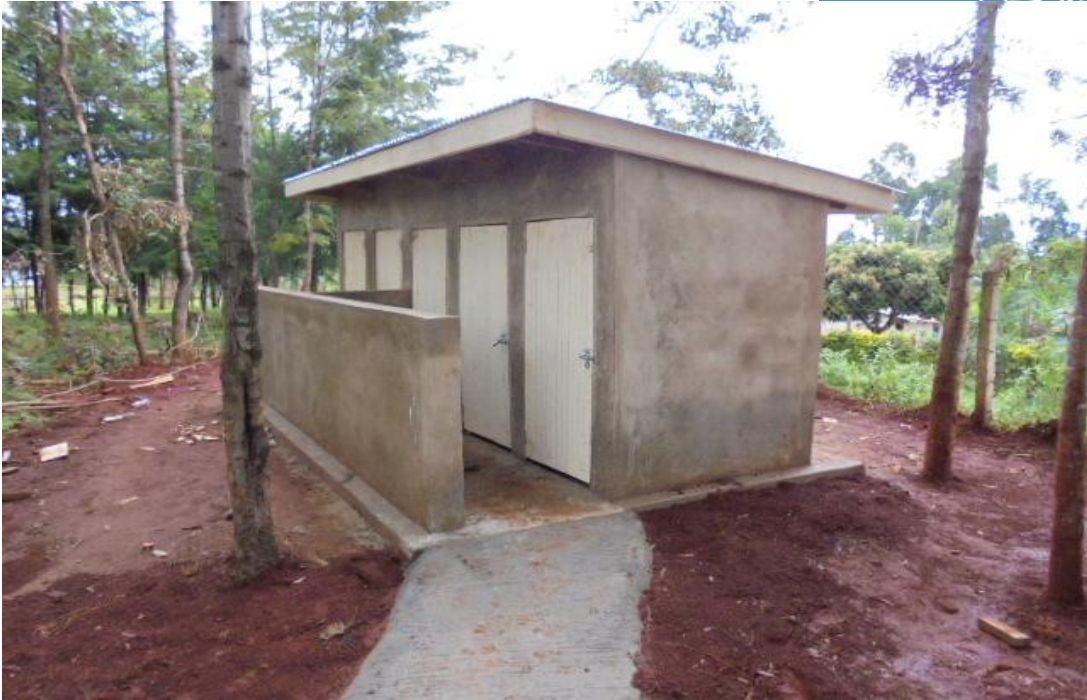
5.0 Ventilated Improved Pit latrines & Bathing hide for Girls at Chanzeywe Vocational Training Center in Mungoma Location, Vihiga Sub-county (Nearing completion—only painting works & branding pending to be done)
