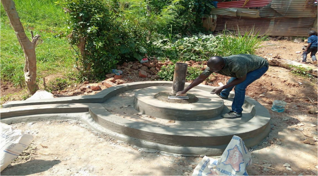
6.0 Completed Anwa/Jiinue Women Group hand dug well in Central Maragoli location, Vihiga sub-county—awaiting solar pump installation
