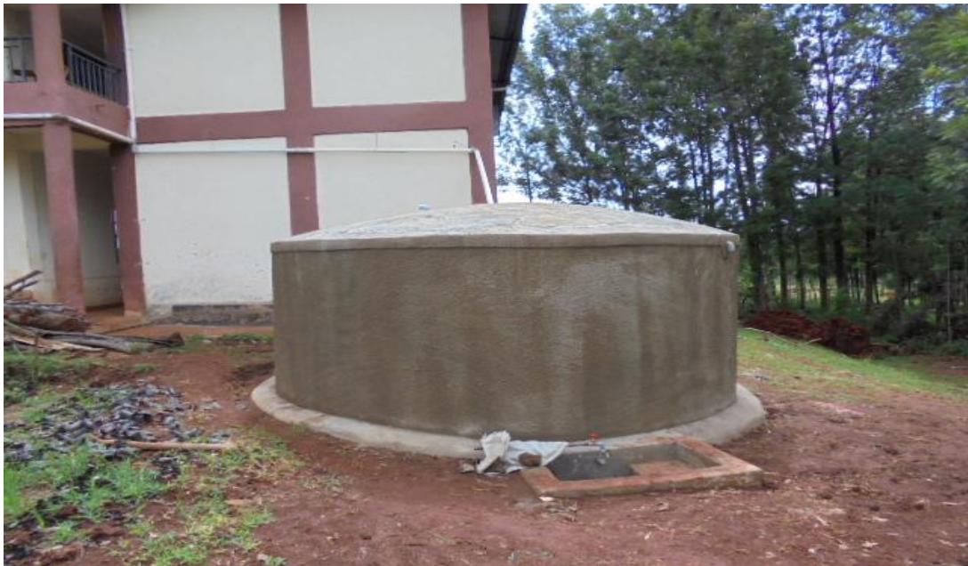
2.0 Completed 30,000litres Ferrous-cement water tank for Chanzeywe Vocational Training Center in Mungoma Location ,Vihiga Sub-county
