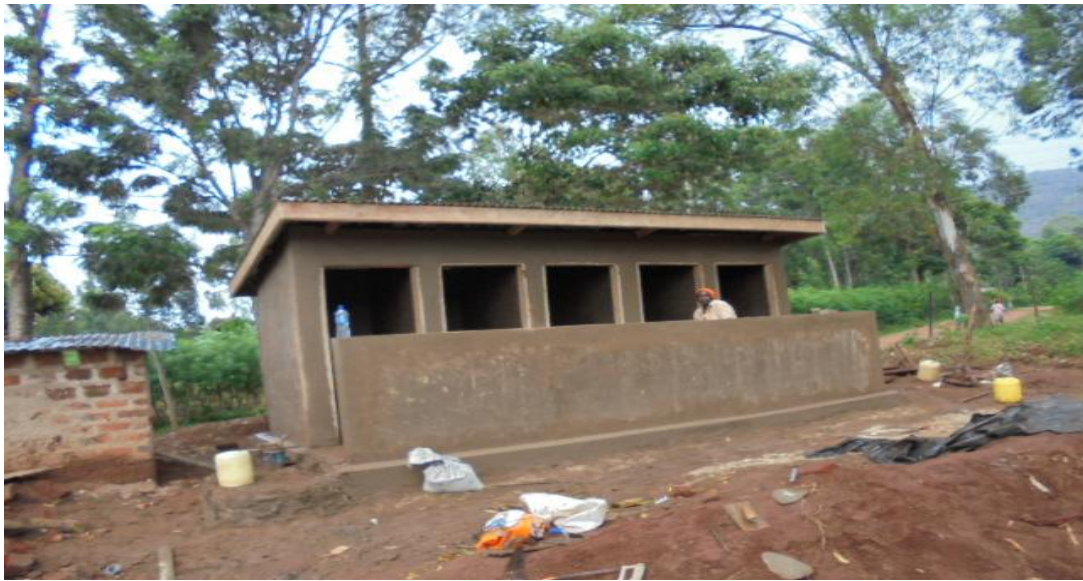
4.0 Ventilated Improved Pit-latrines & bathing hide for Girls under construction for Chandugunyi Primary School in South Maragoli location ,Vihiga Sub-county
