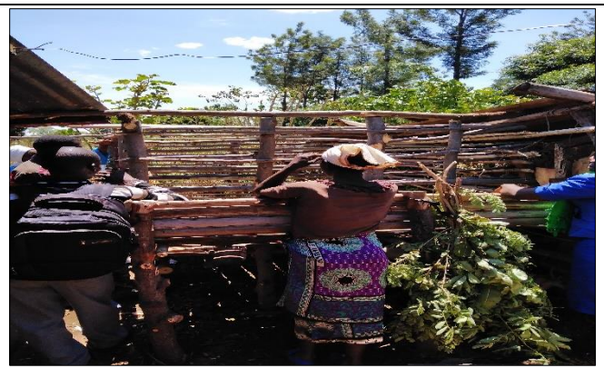
6. Inspection of under construction animal stable/pen for Wendo Mwega women group member
