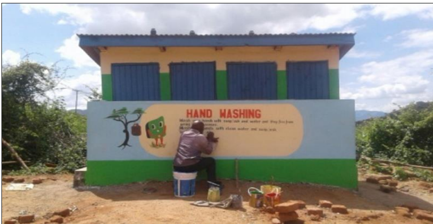
17. Mutuluni Pri. School 2No.VIP Latrines
