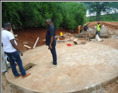
2. Contractor on site discussing work progress with staff at Kaundu secondary school
