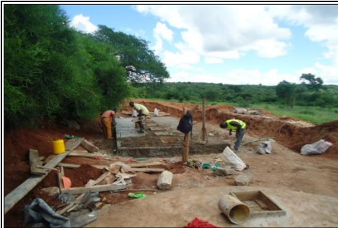
1. Sludge chamber & dome construction works for Biogas production at Kaundu secondary school
