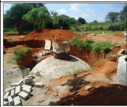
8. Construction works of the dome for biogas production at Kalulini High school
