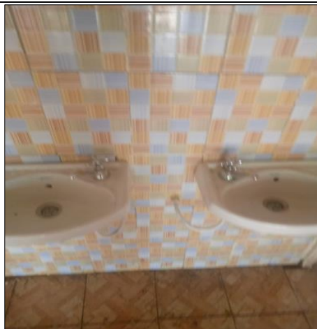
8. Hand washing facilities inside the school latrines
