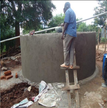
5. Contractor on site ensuring works are done according to specifications at Kaundu secondary school
