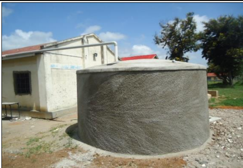
4. 2 nd Completed Ferro-cement water tank of 30,000litres at at Kalulini High school
