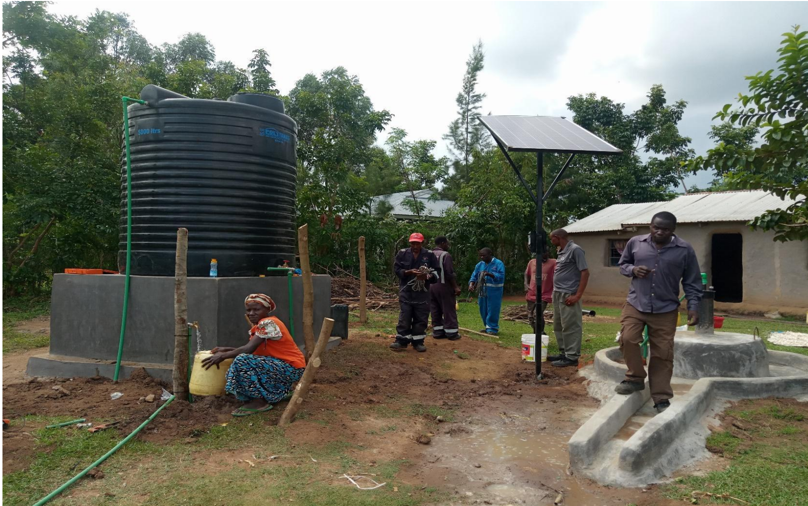
Wapendanao Women Group shallow well installed with Solar pumping system
