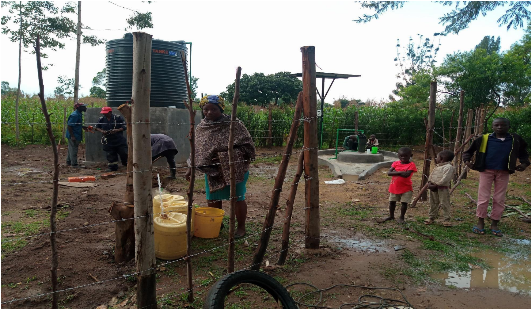
Imani Bora women group shallow well installed with solar pumping system
