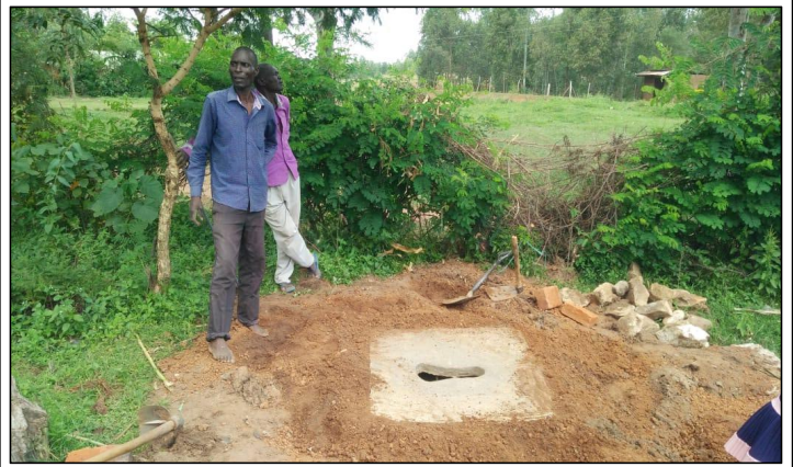
34.0 Mounting of SANPLAT slab on the pit ready for superstructure construction of the Ecosan latrine
