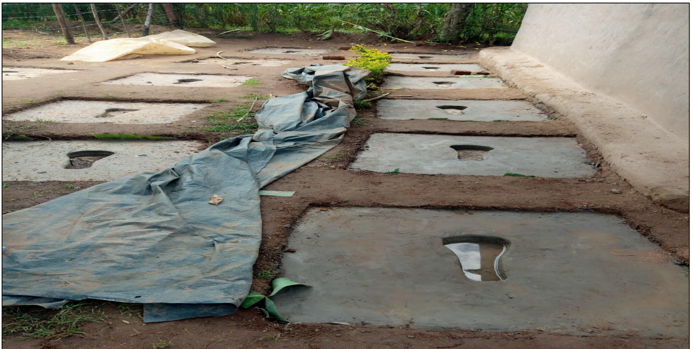
32.0 Slabs manufactured and curing awaiting to be transported to households for SANPLAT Latrine construction & development
