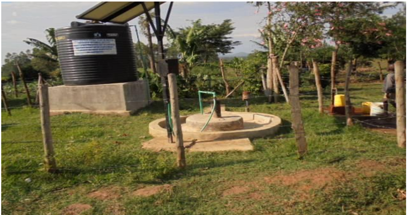
14.0 Completed hand dug well fitted with solar pumping system at Bumula Organic Women Group being used by community members
