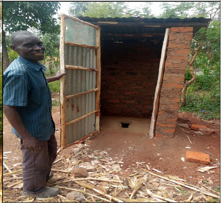
36.0 SANPLAT/Ecosan latrine ready with door and roof fixed ready for use by households
