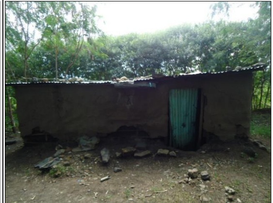
4. Houses destroyed with flood waters in Ongeche village
