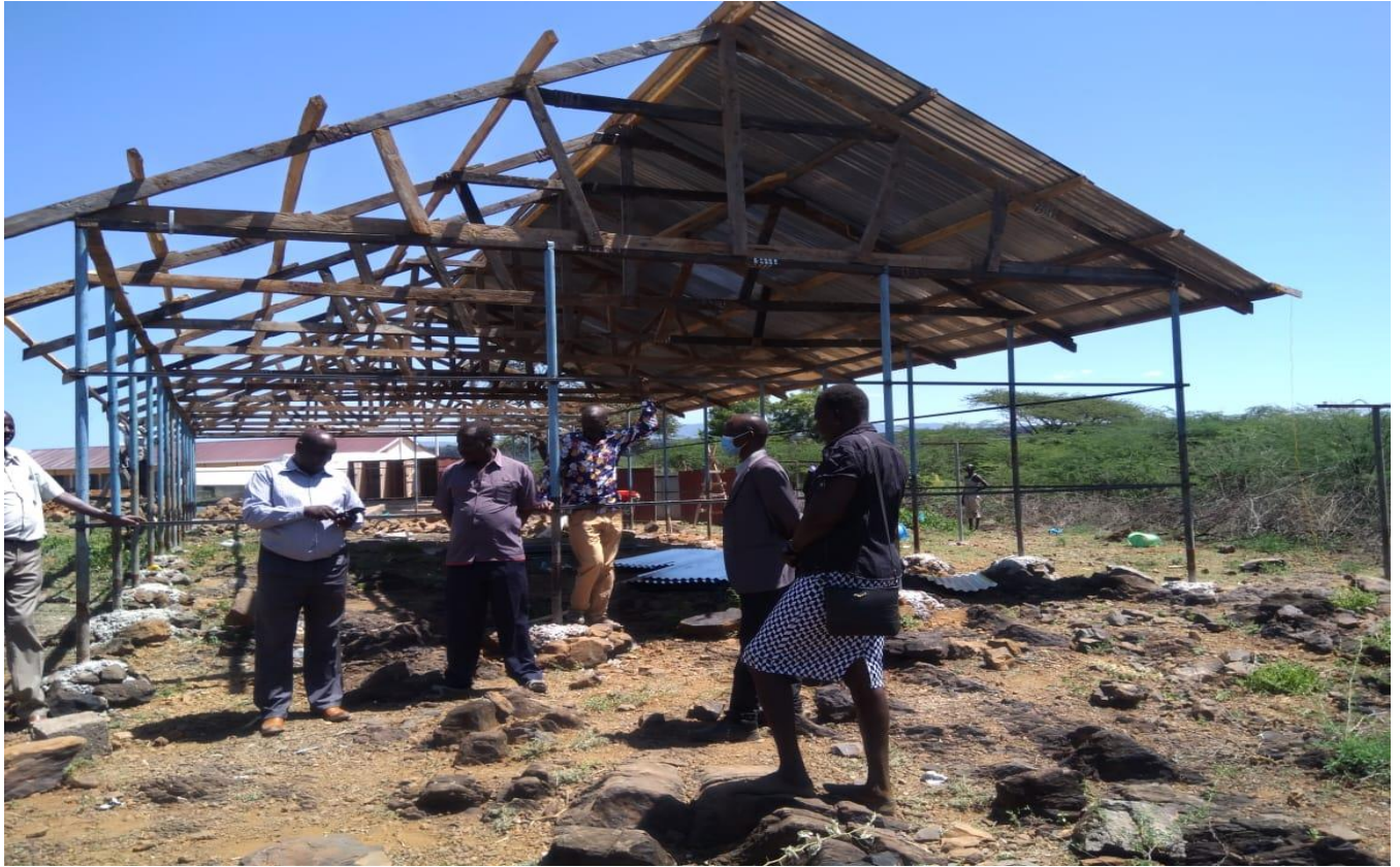
3. Boy's dormitory under construction at Lake Baringo Mixed Secondary school with support of the project
