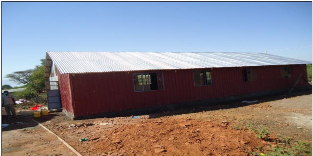
2. Completed Girls dormitory at Lake Baringo Mixed Secondary school with support of the project
